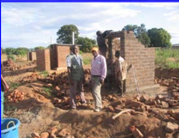
The Head Teacher of Kazembe Basic School and Programs Coordinator posing for the photo next to the VIP Toilets under construction.
